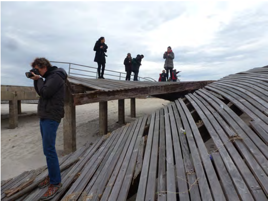
Fig. 8. Photograph of damage in the Rockaways. By Lance Jay Brown
